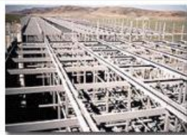
Cooling Tower Structure
