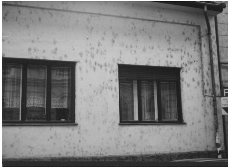
Figure 8: Plastered Façade in the Polluted Air
