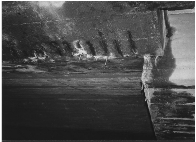
Figure 9: Stalactite Creation on the Reinforced Concrete
