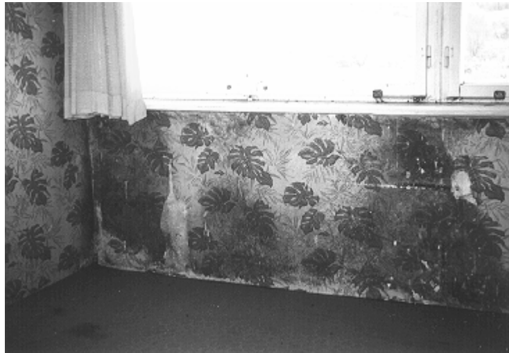
Figure 5. Mildew traces on the facade wall
