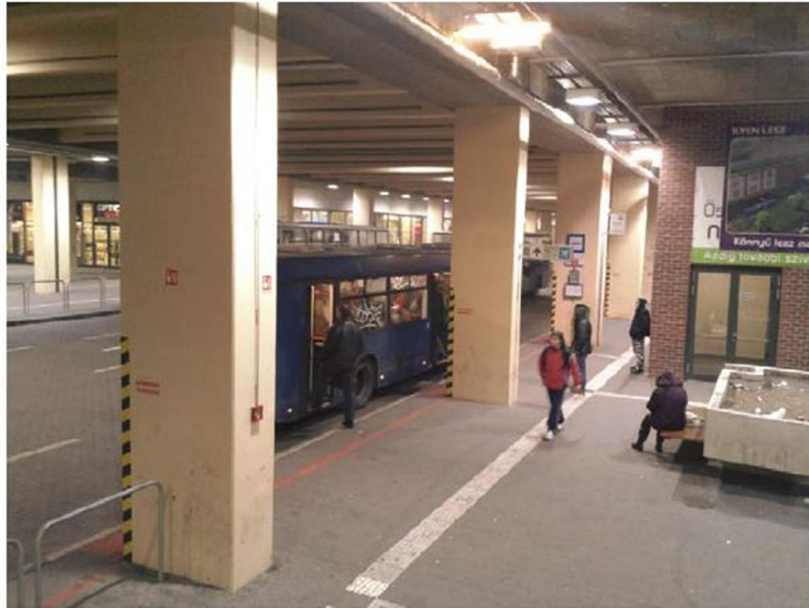
Figure 19: Example of design faults
