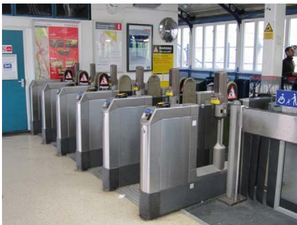
The gate line barriers, which are operational during peak hours
