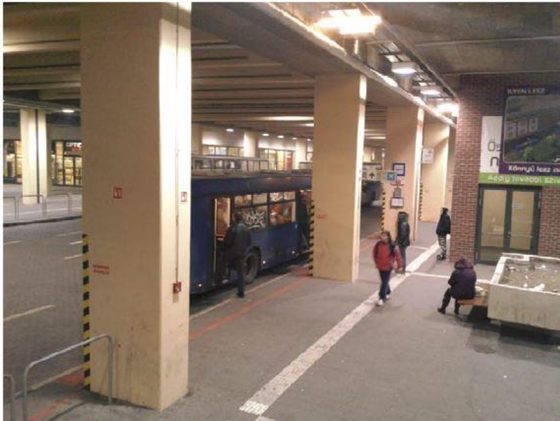
Figure 19: Example of design faults
